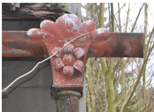
Fig. 14.: Bublava house No. 129 – detail of rainwater downpipes. [Source: Dominika Výšková (photograph), 2024].
