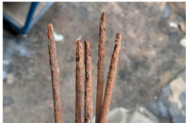
Fig. 2: Fragments of corroded prestressed tendons
