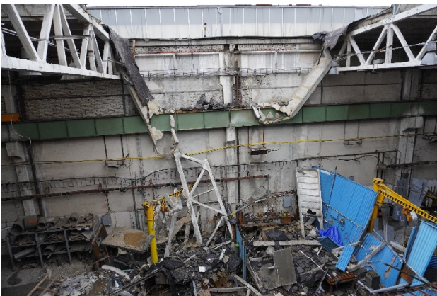
Fig. 1: Collapsed roof structure - December 2023, Czech Republic
