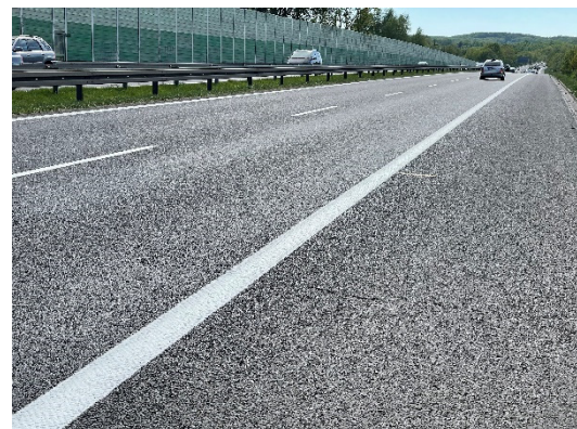
Fig. 2: View of an example of a transverse crack in the A6 motorway pavement after 17 years of service
